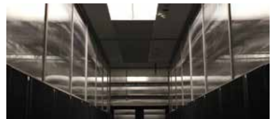
Cabinet Supported Hot Aisle Containment
