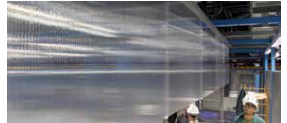
Ceiling Supported Hot Aisle Containment
